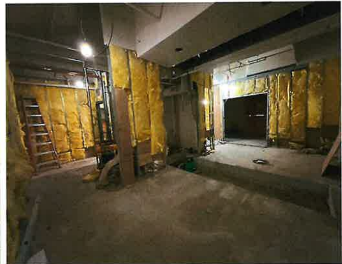
Annex Bathroom Underground Plumbing
