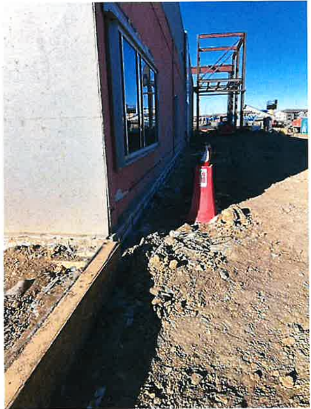
Corner of south addition and steel at new entry on east side of building.
